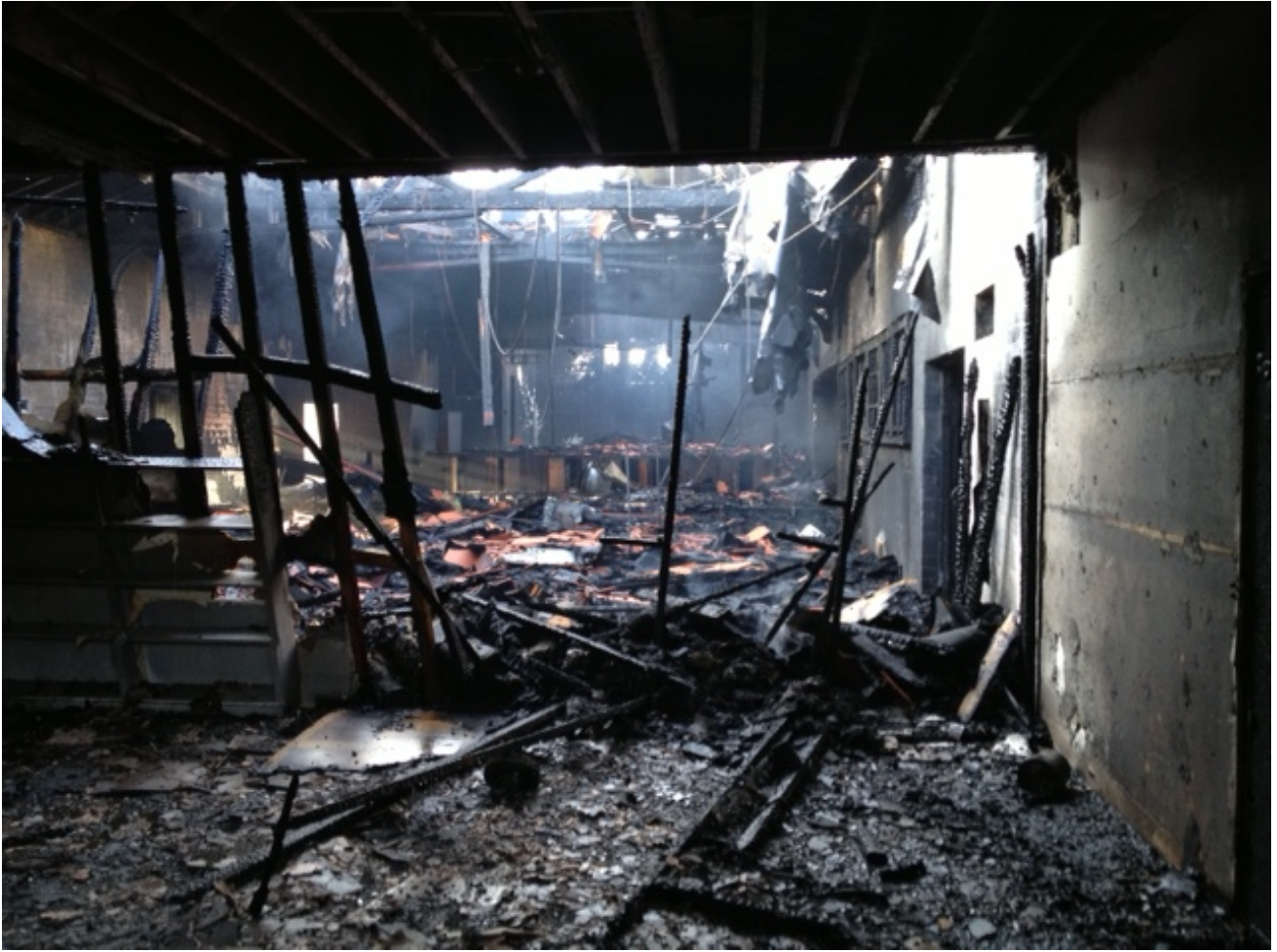
Church Interior, following the fire
